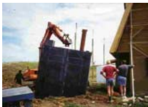
Figure 1 Ozeki septic tank to change any organic inputs into bio-gas
