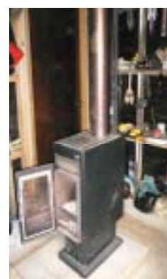
Fig.6 Solar panels in the above and the wet back in the shed to make hot water
