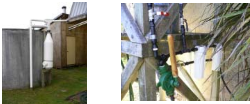
Rain water tank and sludge trap
